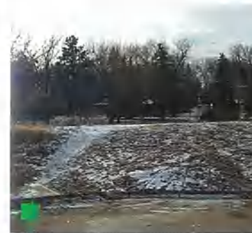
Informal access paths worn in dyke slopes
